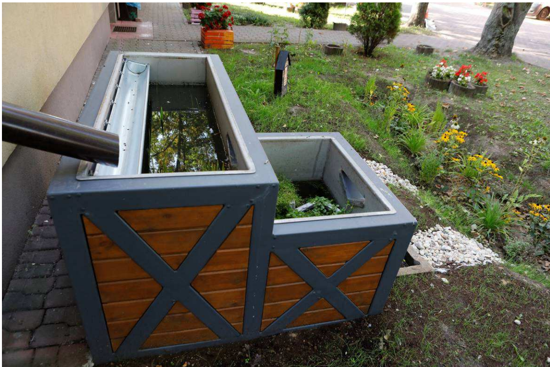
Photo 32 State of the site after the works - Climabox and swale + insect house
