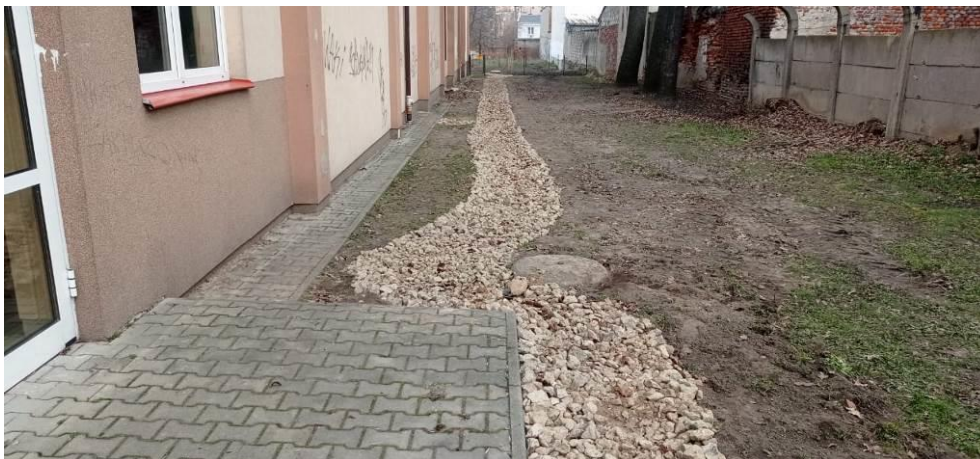
Photo 8 Appearance of the site after completion of the works - dry streams collecting water from downspouts and directing it to the Climapond
