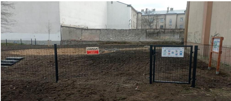
Photo 5 Appearance of the site after completion of the works -Climapond with educational boards
