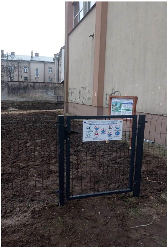
Photo 10 Appearance of the site after completion of the works -Climapond with educational boards
