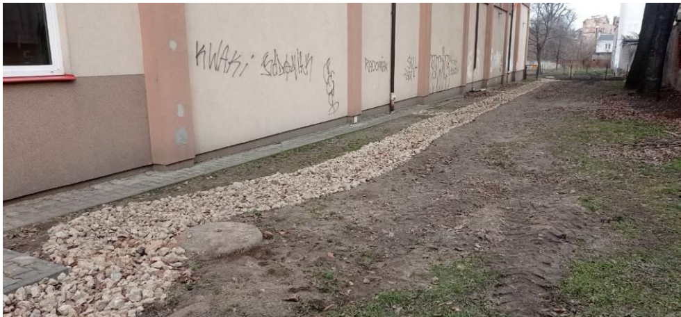
Photo 9 Appearance of the site after completion of the works -Climapond with educational boards
