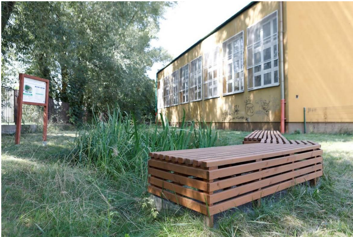
Photo 11 Appearance of the site after the works - Climapond with bench + information board
