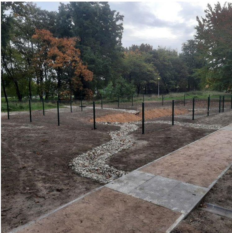
Figure 8 Appearance of the site after completion of works – Climapond, dry streams and culvert under the pavement - permeable surface
