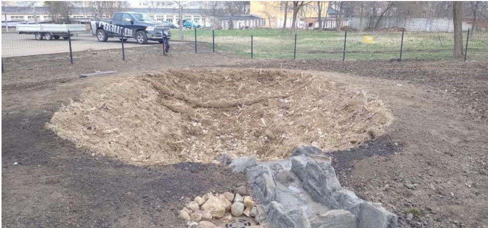
Photo 11 Appearance of the site after completion of the works -Climapond with a water dispersal element made of plastic imitating natural stone; Climapond slopes lined with coconut mat to hold aquatic vegetation
