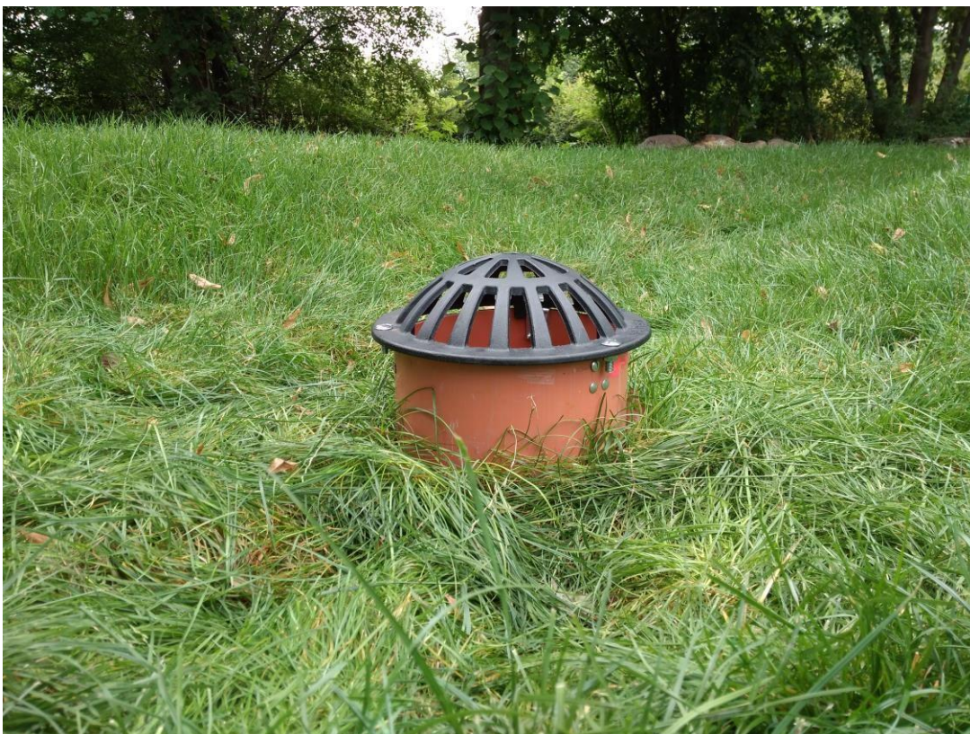
Photo 12 Appearance of the site after the works -emergency overflow to the sewage system by Climapond
