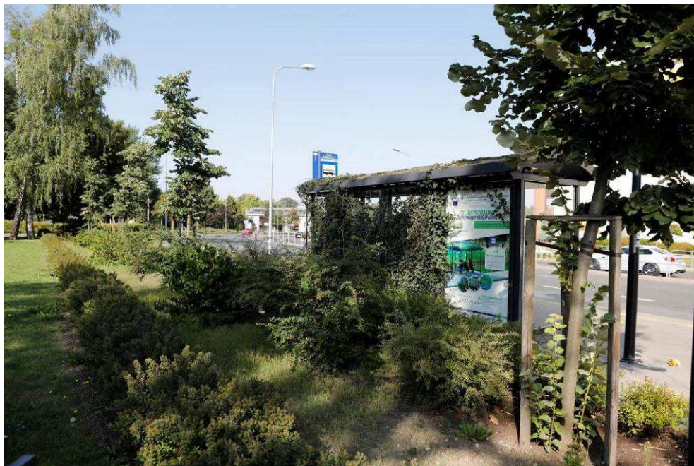
Photo 8 State of the site after the works - Green Bus Shelter with Green Roof and Green Wall - planting of plants
