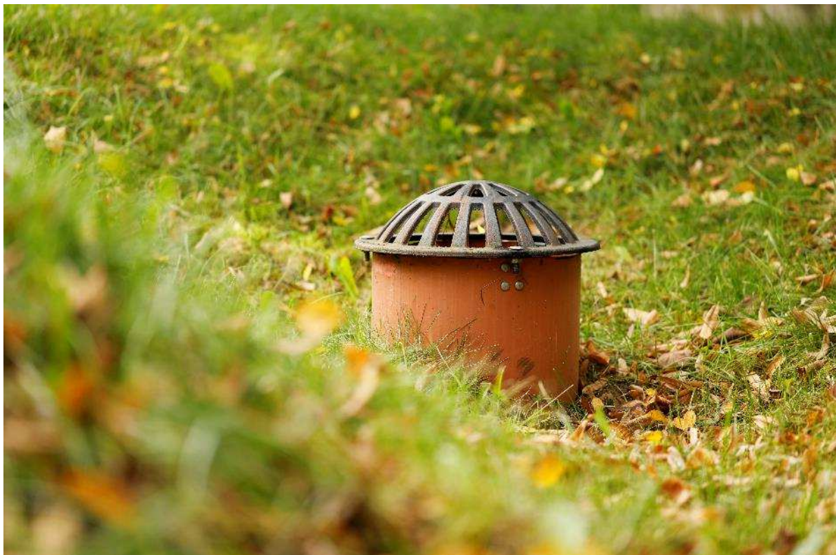
Photo 2 Appearance of the place after completion of works - Emergency overflow in the middle of the basin
