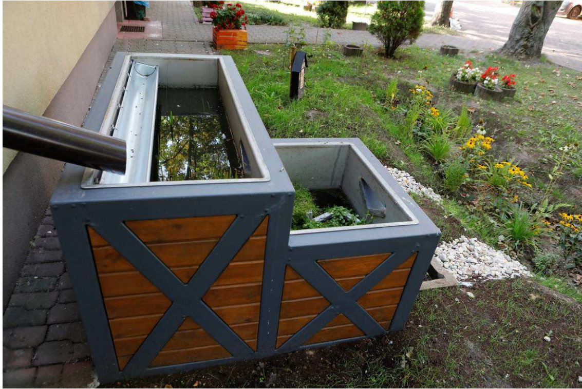
Picture 25 Appearance of the site after the construction- Climabox + Swale + house for insects
