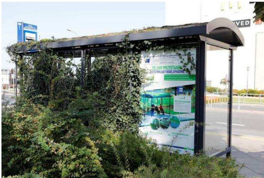
Photo352 Appearance of the site after the construction- Rain garden in the basin behind the shelter
