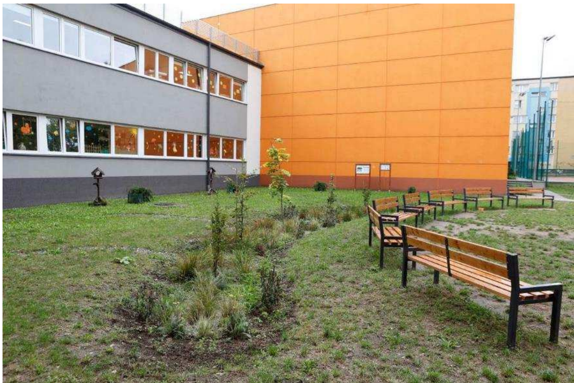
Picture 6 Appearance of the area after the construction- Swale with a row of trees + elements of small architecture
